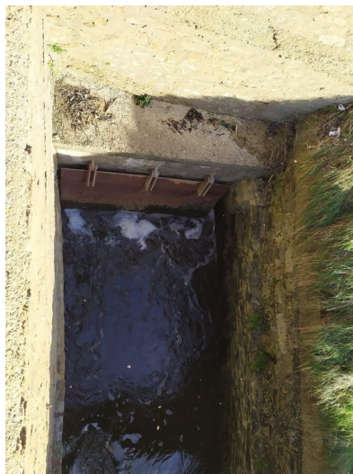
Figure 8: Clapets sur la digue (C. ROSSIGNOL)
